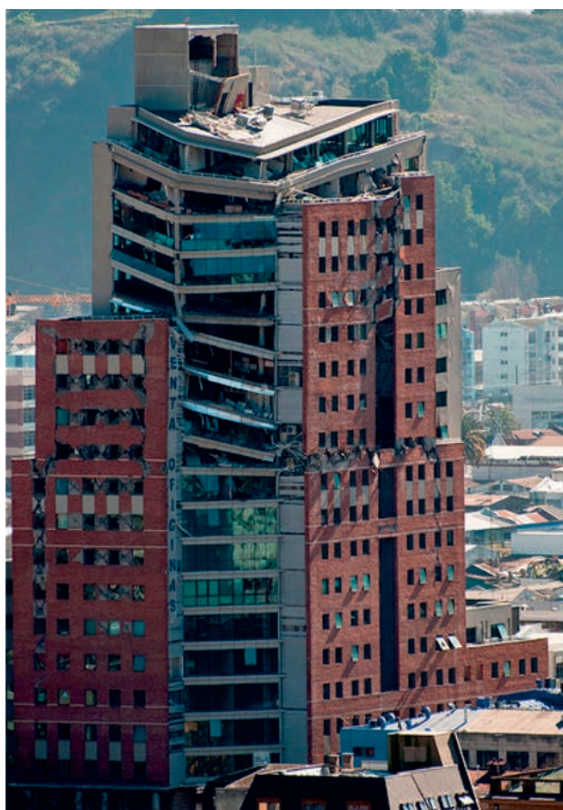
Prăbușirea clădirii Torre O'Higgins, Chile, 2010 (sursa: http://www.flickr.com/photos/janotrix/4877345252/ )
